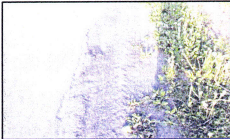
Fletcher Chapel Road shoulder condition
