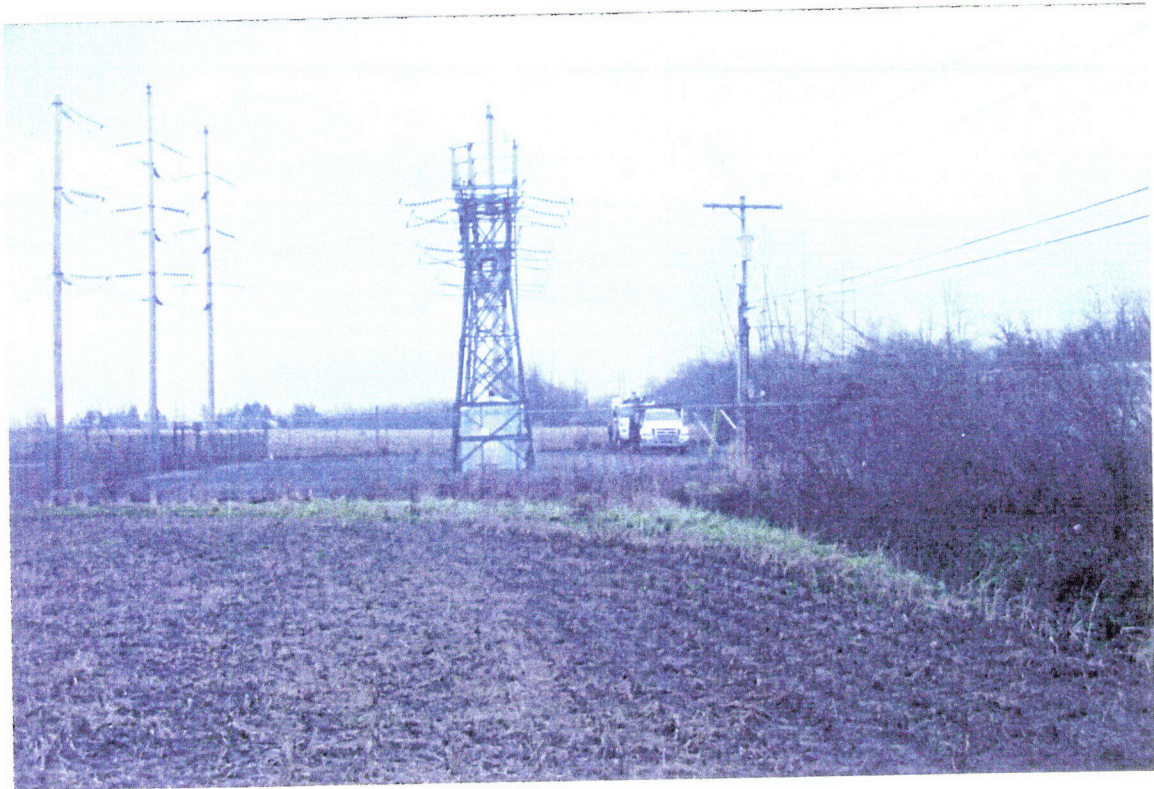
Photograph 21 Substation at Southeastern Corner (Project Area) Looking West
